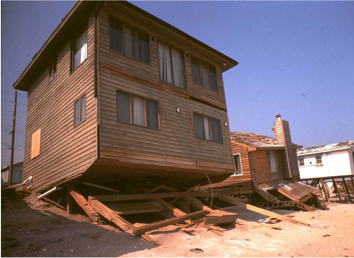
Figure 3: Short piling foundation failures (Class 1b) on high-elevation shoreline (Type A). Location: Kure Beach NC after Hurricane Fran.
