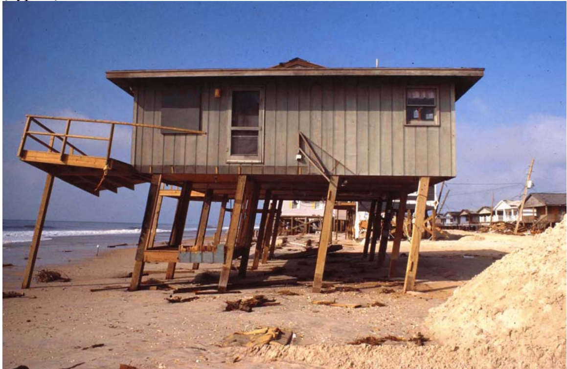
Figure 4: Short piling foundation (Class 1b) near failure on low-elevation shoreline (Type B). Location: Surf City NC after Hurricane Fran.
